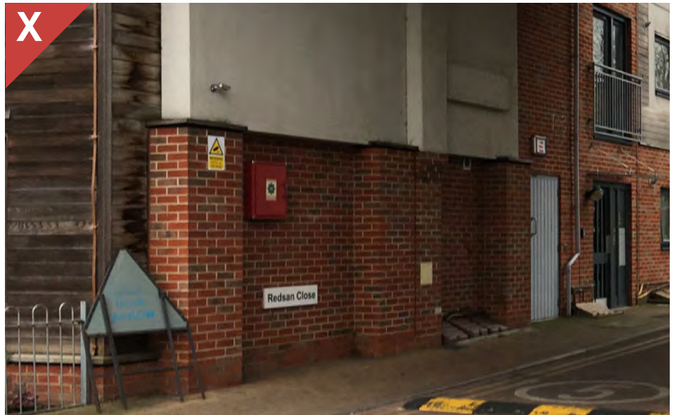
Figure 2.27a: Poorly coordinated placement of visible ancillary items on elevation visible from the street has a negative impact on the building's appearance.
