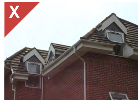
Figure 2.19h: Poorly proportioned and positioned dormers and eaves results in a poorly resolved roof.
