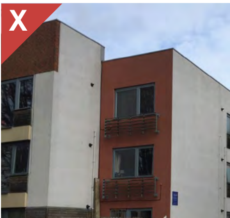
Figure 2.23j: The change in render colour at the corner contributes to a flimsy appearance, highlighting that it is surface applied and lacks depth.
