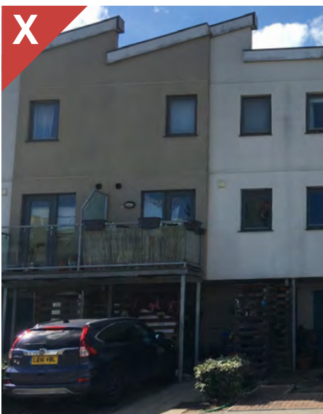
Figure 2.26a: External balconies with supports that are not integrated into design of the proposal. The use of glass balustrades have resulted in occupiers retrofitting screening devices to provide privacy that exacerbates the poor appearance.
